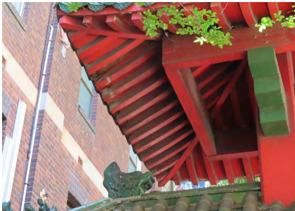
Figure 4.16 Evidence of plywood delaminating from the underside of the curved upper roof of the eastern bay.
