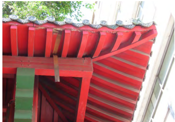
Figure 4.17 Underside of upper roof on the western bay with deteriorated, delaminating plywood soffit.
