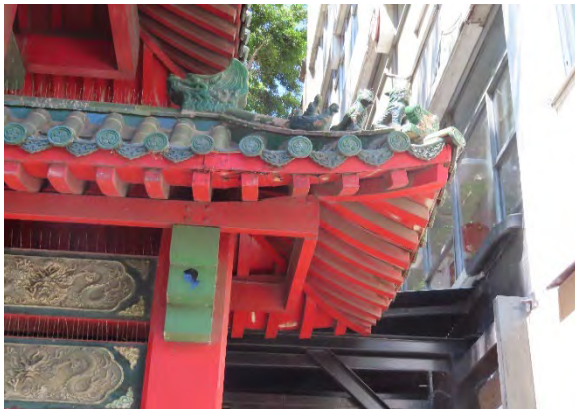
Figure 4.18 Missing/broken ceramic tile on the lower roof—western bay.
