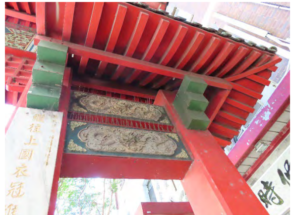
Figure 4.11 Underside of curved timber rafters and plywood soffit on the lower roof.
